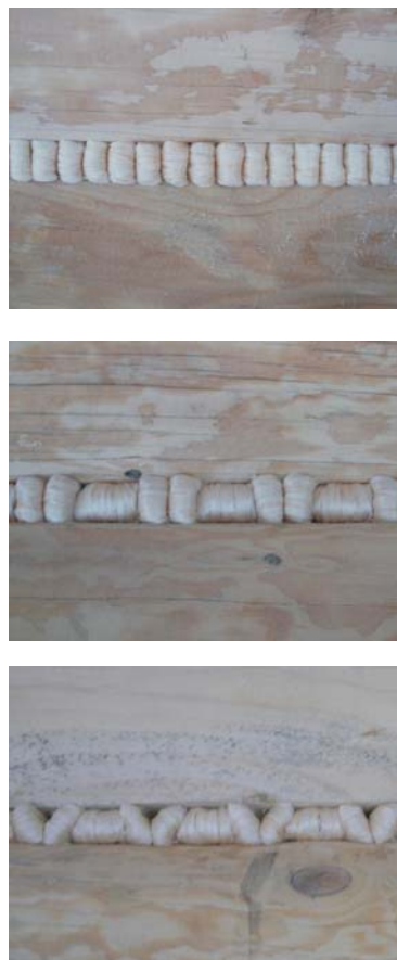
Rys. 2. Wzory wełnionki zwijane i wbijane w szczeliny między balami Fig. 2. Specially planed chips, curl up and stick in the cracks between the logs
